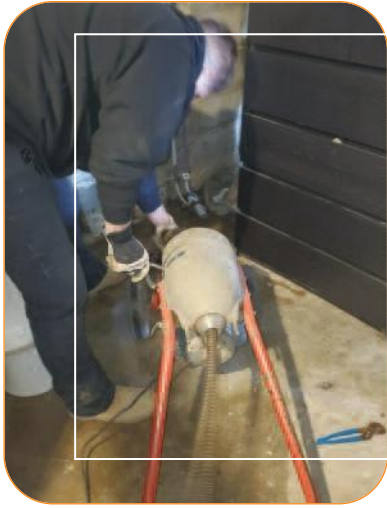
John Oakes, All Pro Plumbing, works to remove a residential sewer clog.
