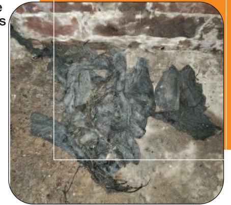
Flushable wipes that were removed from a sewer line.
